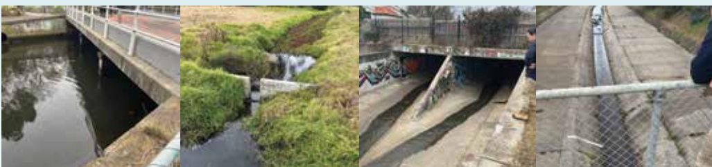
Site inspection for new sensor deployment in Melbourne (Elster catchment-above ground)- 8 July.
