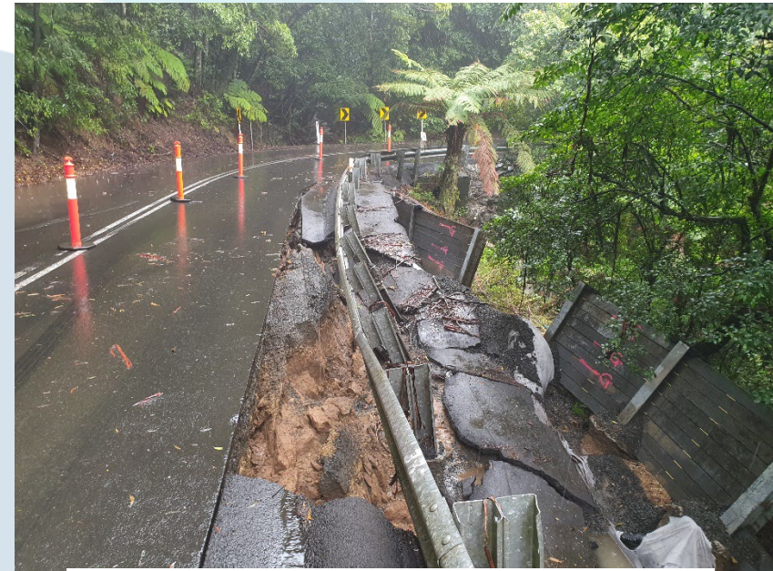
Jamberoo Mountain Road Failure, NSW 2020.
