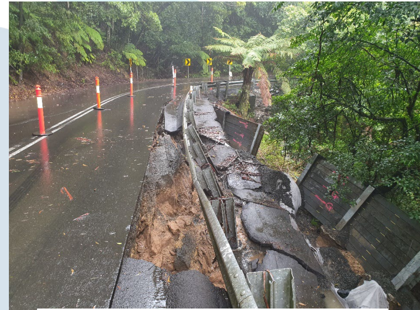
Jamberoo Mountain Road Failure, NSW 2020.
