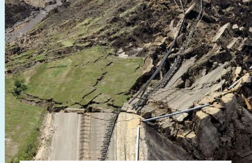
Failure of Yallourn East Field Mine, VIC 2007.
